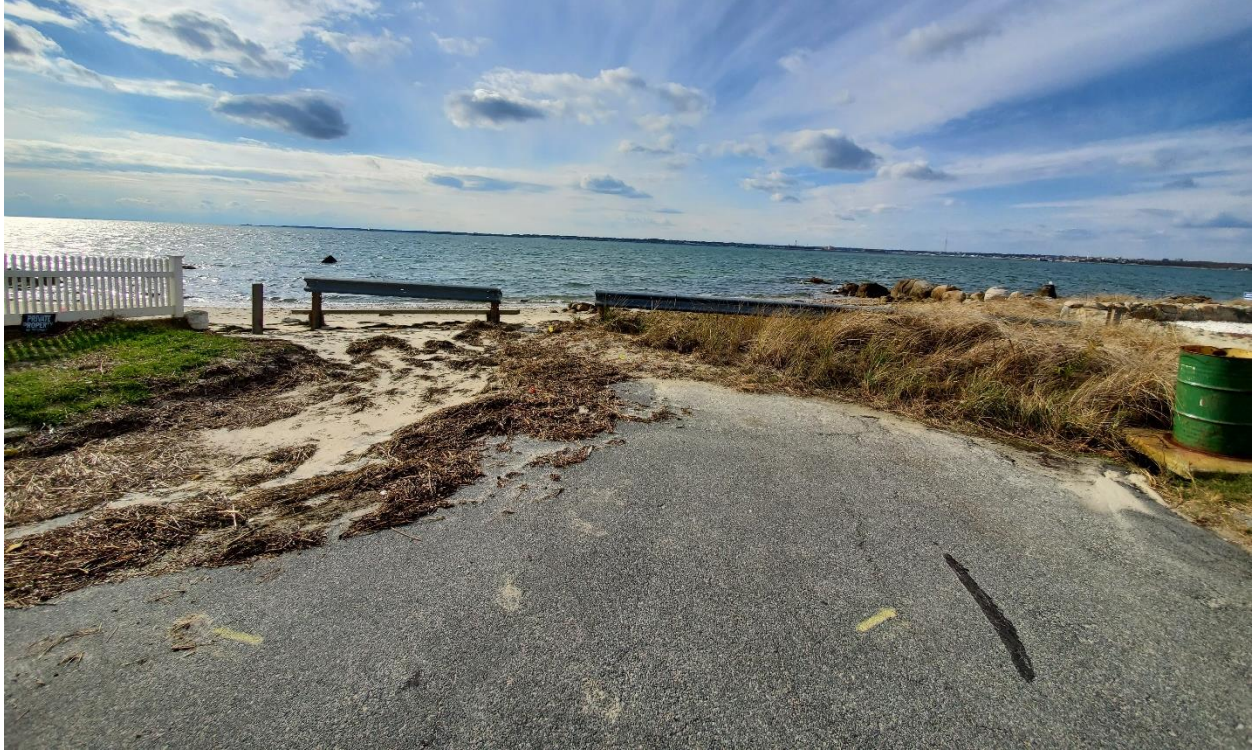
Photo 8. View of the end of Jerusalem Road (facing west) where the majority of work within jurisdictional areas will occur. A portion of the pavement will be removed to allow for the construction of a bioretention area, and approximately 2,900 SF of this area will be restored with native plantings.
