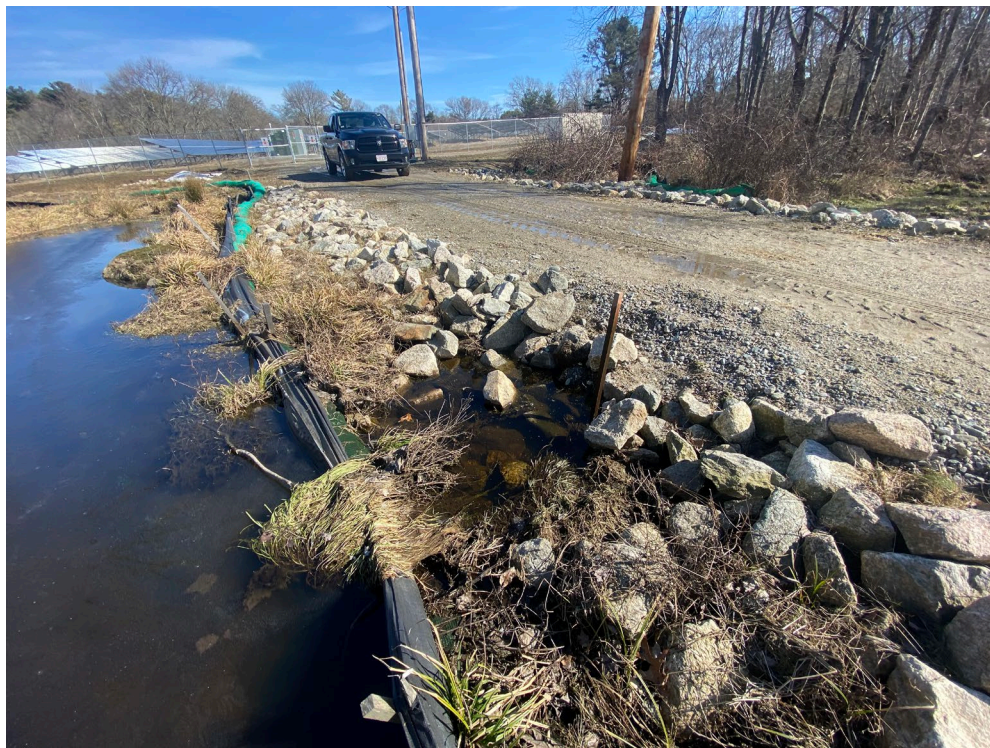
Figure 6: Rip-Rap Failure at North End of Wetland Crossing "A"
