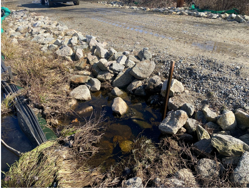
Figure 7: Rip-Rap Failure at North End of Wetland Crossing "A"
