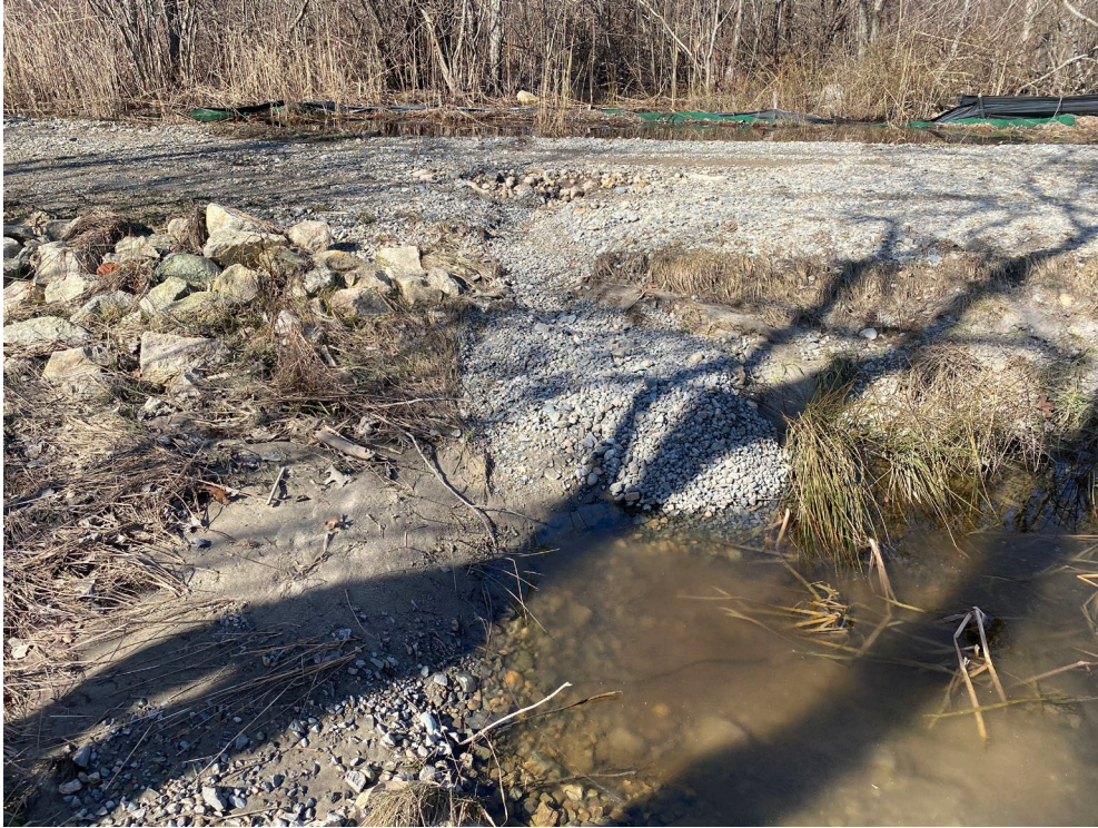
Figure 3: Rip-Rap Failure East of Wetland Crossing “B” at Southern Swale
