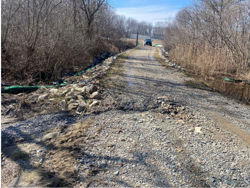
Figure 1: Rip-Rap and Roadway Failure East of Wetland Crossing “B”
