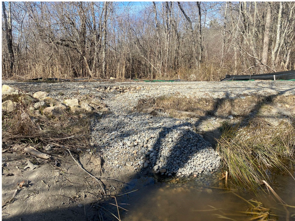
Figure 4: Rip-Rap Failure East of Wetland Crossing “B” at Southern Swale
