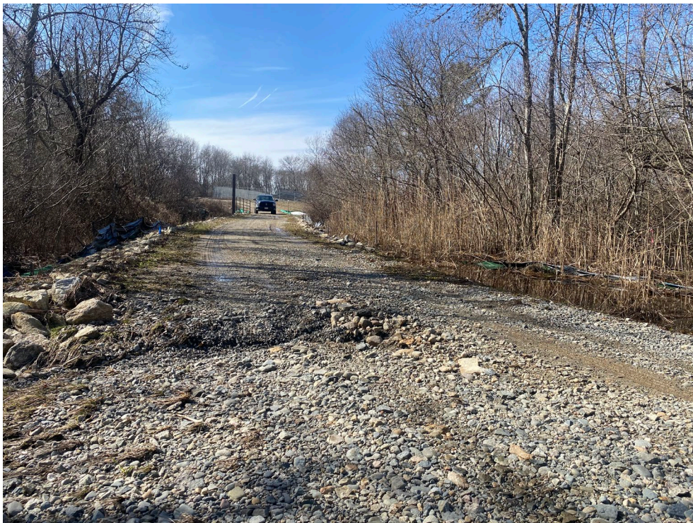
Figure 2: Rip-Rap and Roadway Failure East of Wetland Crossing “B”
