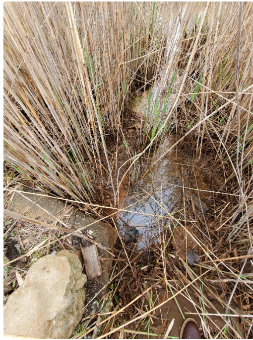
View of culvert/outlet pipe from western portion of the wetland to abutting landfill drainage swale
