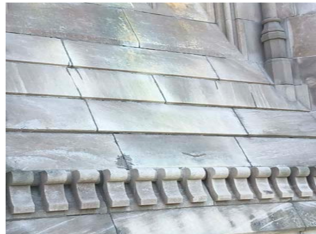
Shingle stone sills have open joints causing water infiltration.
