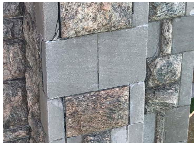
Cracks at buttress stone.
