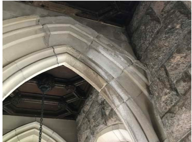
Eroded stones at interior of porch arches.
