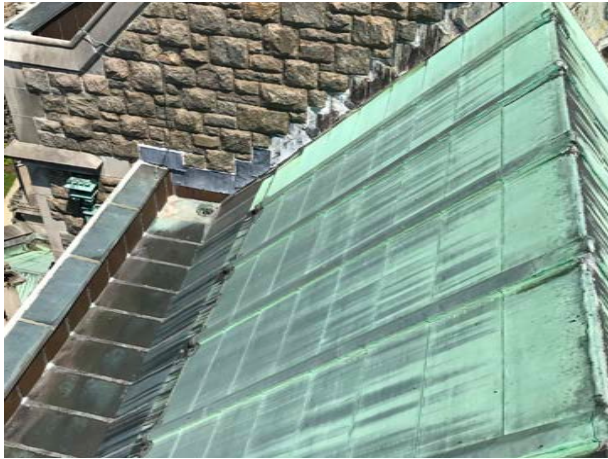
Older copper roofing with numerous patches over choir at west end of building.
