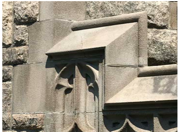
Cracked stones at parapet above porch.
