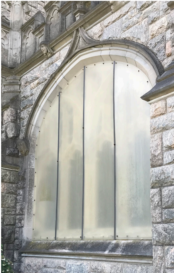
Yellowed Plexi-glas security panels at the cloister should be replaced with material and methods to improve aesthetics while maintaining security
