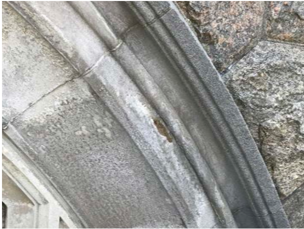
Frost-damaged trim stone.
