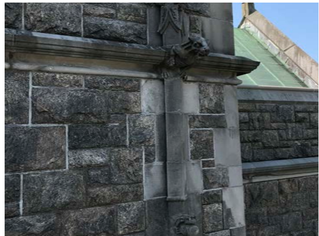
Open mortar joints.
