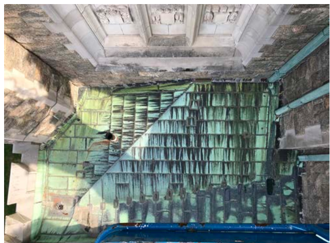
Older copper roof at southwest corner with numerous patches and open joints in solder.
