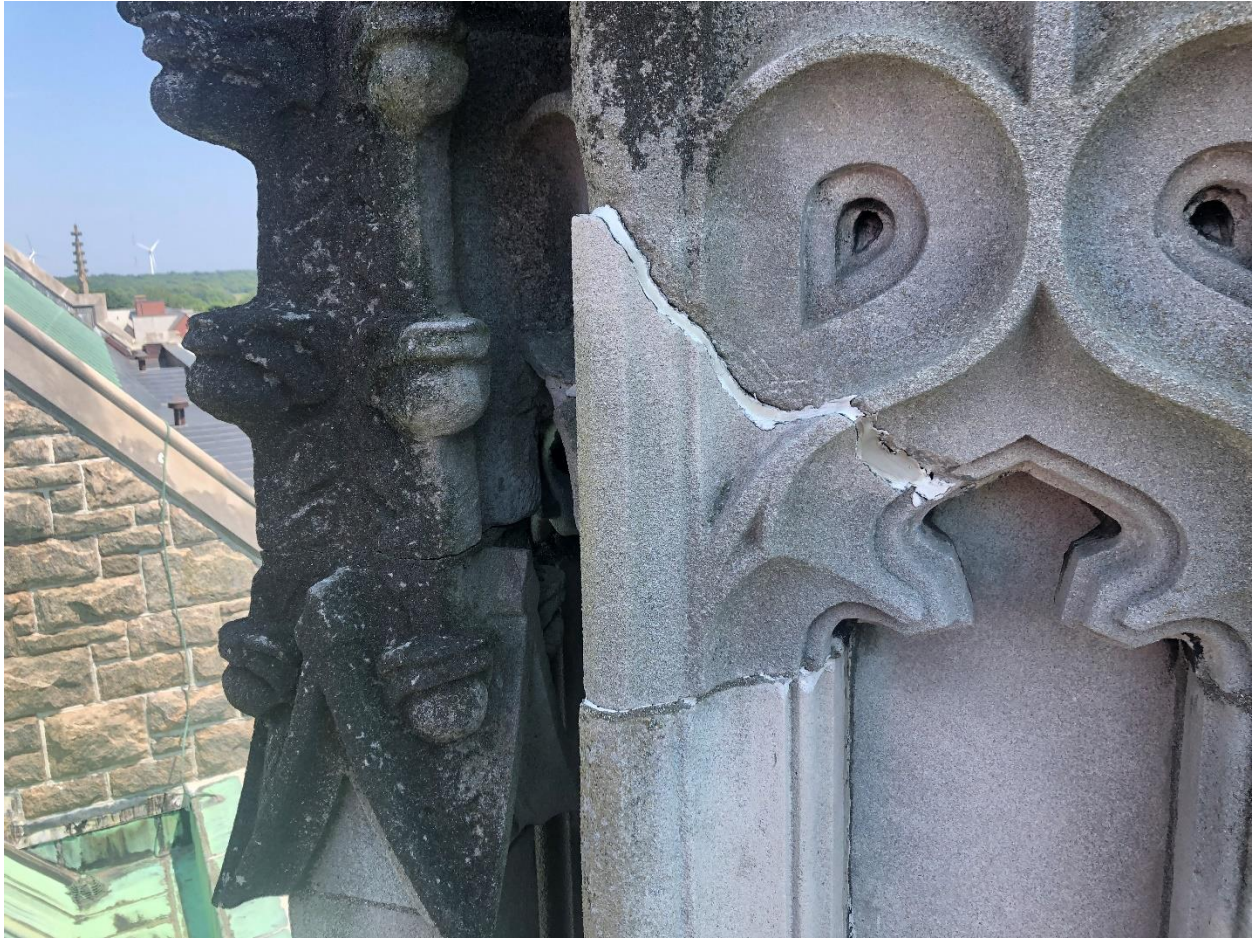
The large pinnacle on the southside of the west elevation was damaged by lightning and repaired with sealants. The repairs have reached the end of their service life. The cracked fragments have to be removed and reattached with an exterior rated stone epoxy.
