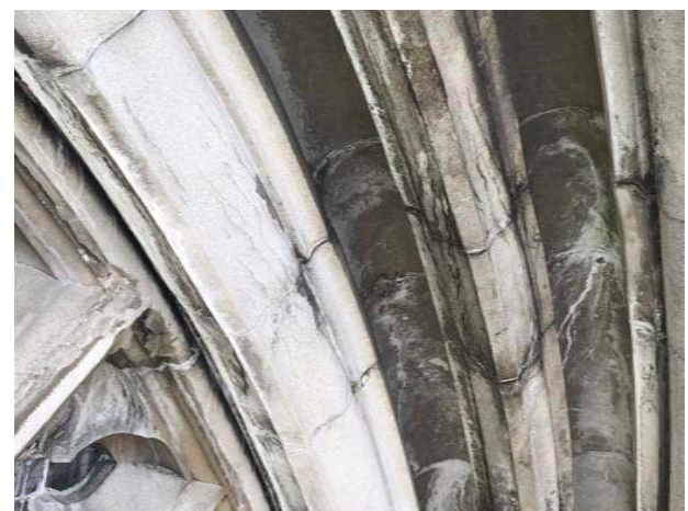
Deteriorated stone at arch over main window is evidence of water infiltration and movement of stone.
