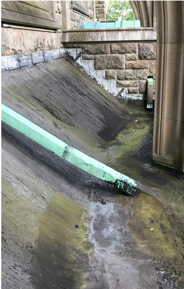
Downspouts from the nave roof drop to the aisle roof then enter the building briefly to then go to external collector boxes.
