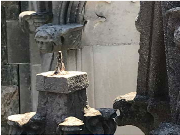
At the south side of the west elevation, the inspection team removed a precarious finial.
