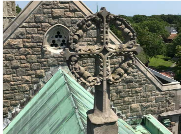
Cross at peak of roof is loose and cracked.
