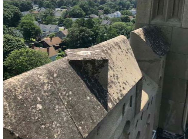
Evidence that there may have originally been finials here at all four elevations.
