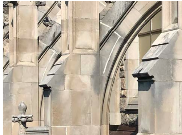
Arch stones at the flying buttresses have slipped due to movement and require pinning to stabilize the stones.
