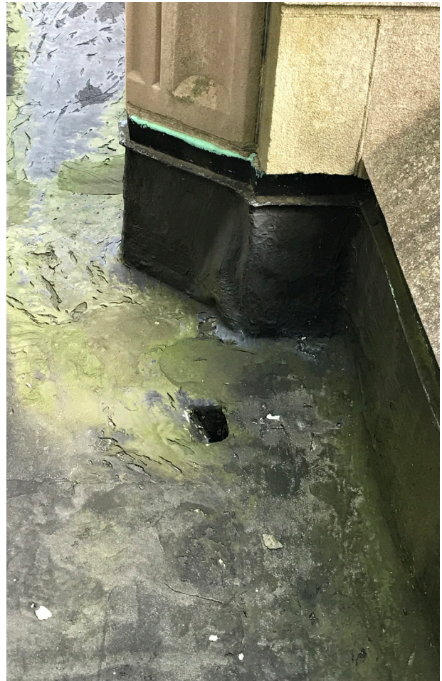
Rain leaders enter the building and are the suspected cause of interior damage.
