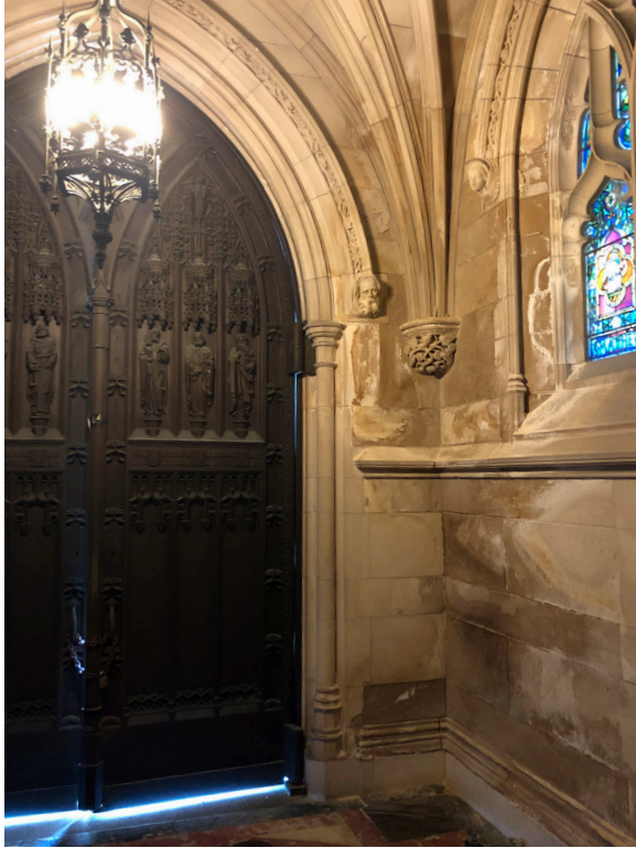
Moisture effects on southwest entry portico. The moisture issues at the building's interior sweep from the east window around the south side and through the choir to the northwest corner. All areas show the effects of moisture penetration that has caused leaching of colored oxides, rust, and other materials.
