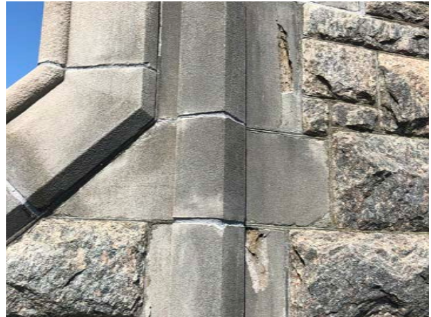
Spalled limestone at gable coping.
