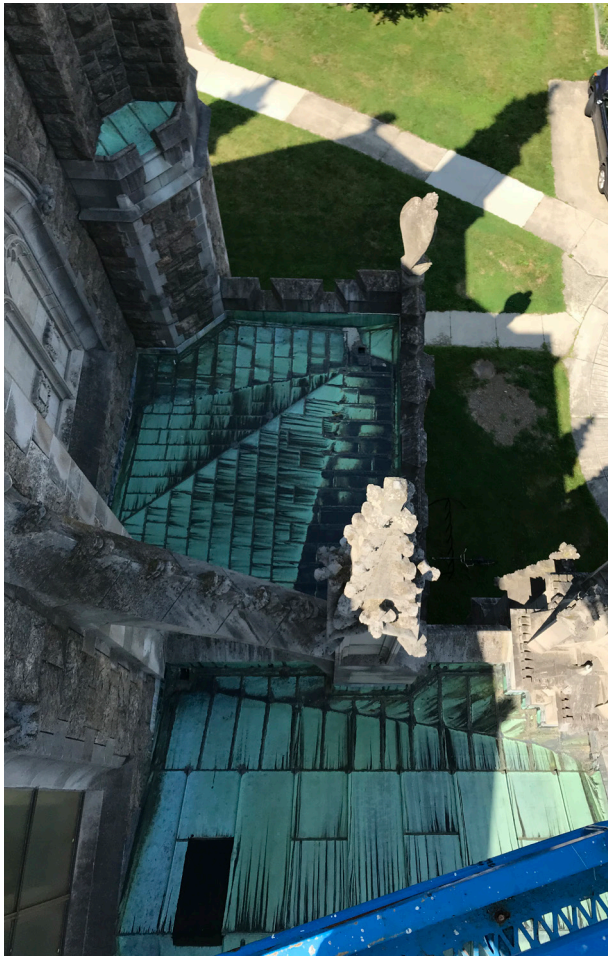
Original copper roof beyond its life expectancy at northeast corner.
