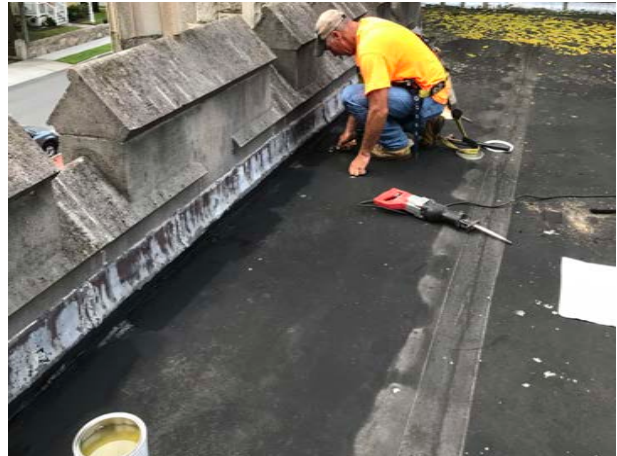
Current roof is .060 EPDM applied on top of 4-ply bitumen roof on plywood. During August 2019 assessment a number of holes in the EPDM were patched.
