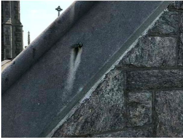
Failed caulk at gable coping. Note: This caulk contains asbestos.
