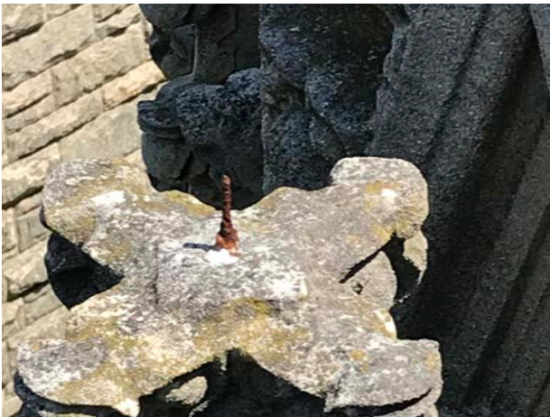
Lost and cracked finials due to corroded steel pins at north side of west elevation.
