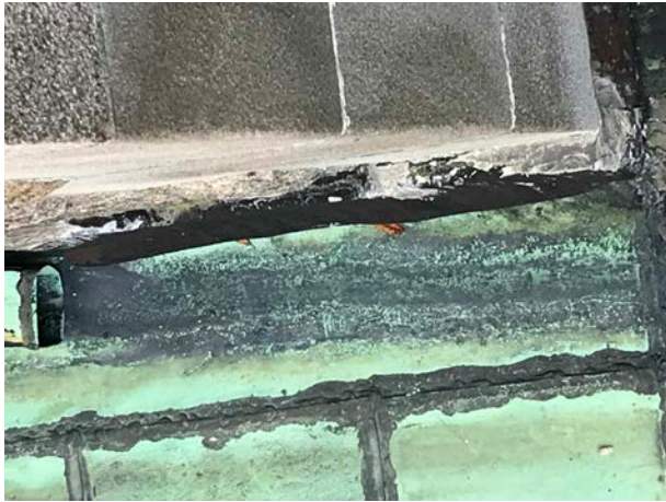
Detailed view at southeast corner roof shows many campaigns of repairs to open seams with mastic.
