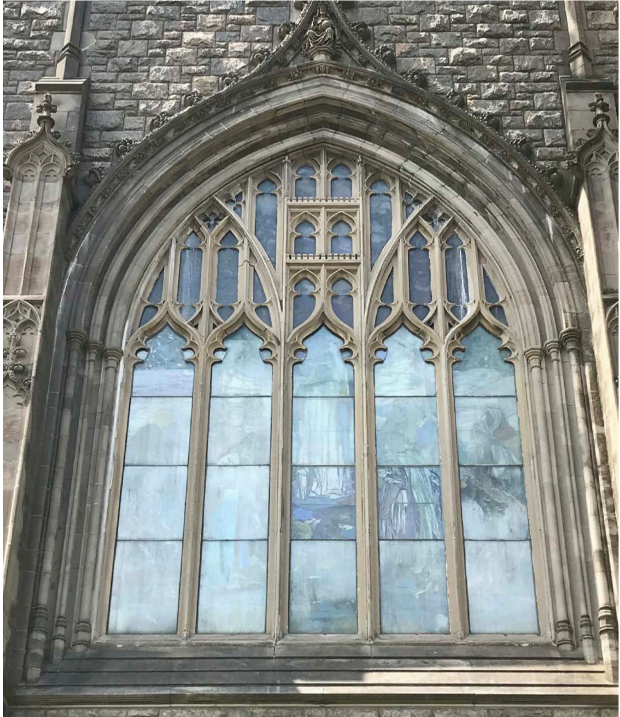
East window that has benefited from Plexi-glas removal during the lift inspection to allow original glass's beauty to be visible and also remove a condition that is causing excess moisture against the glass. The outermost layer of the original glass (visible here) is a ripple texture.
