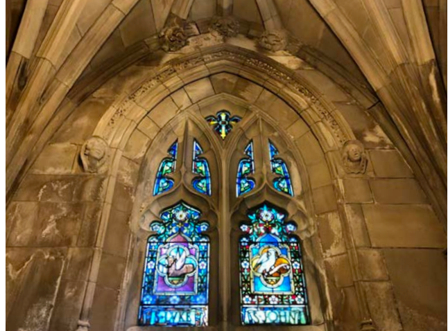
Southwest entry portico moisture effects.
