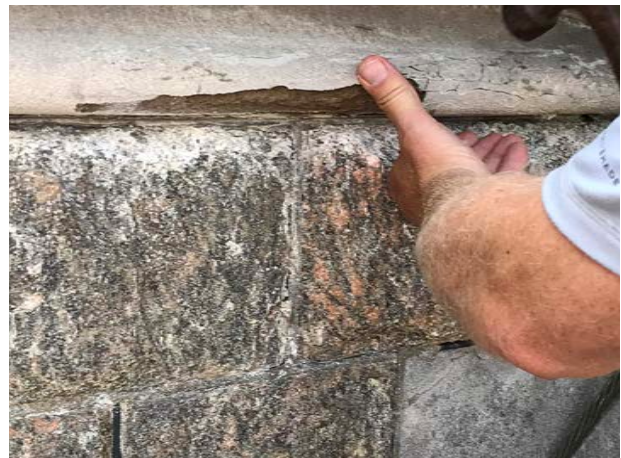
Frost-damaged trim stone.
