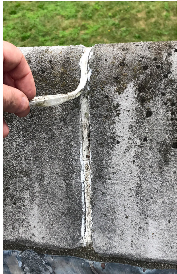
Caulking at coping stones has failed. Note that the caulking has tested positive for asbestos.
