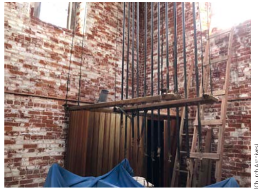
The bell ringing room has extensive deterioration of the walls due to moisture infiltration.
