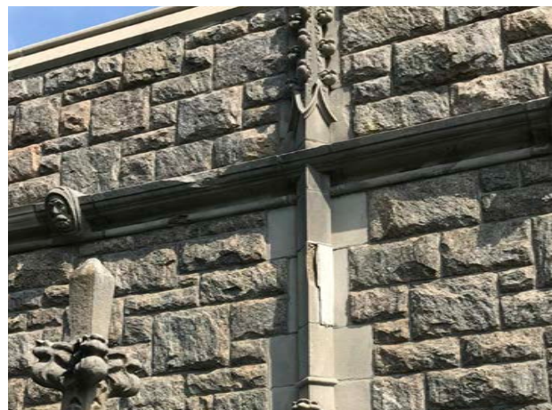
Deteriorated and broken stone.
