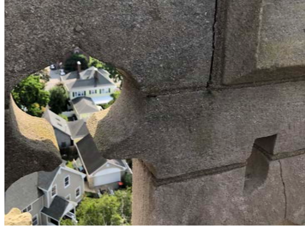
There are many open joints and cracks in limestone tracery parapet above the tower roof.
