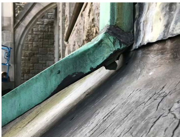
Elbows at downspouts have blown out from freeze-thaw cycles and copper is beyond its expected life.
