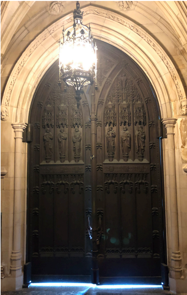
Existing bronze doors are difficult to operate due to a combination of factors: A slipped arch stone, a compressed rubber shim at the hinge, and perhaps an undersized pintel hinge. See Structural Assessment on page 79.
