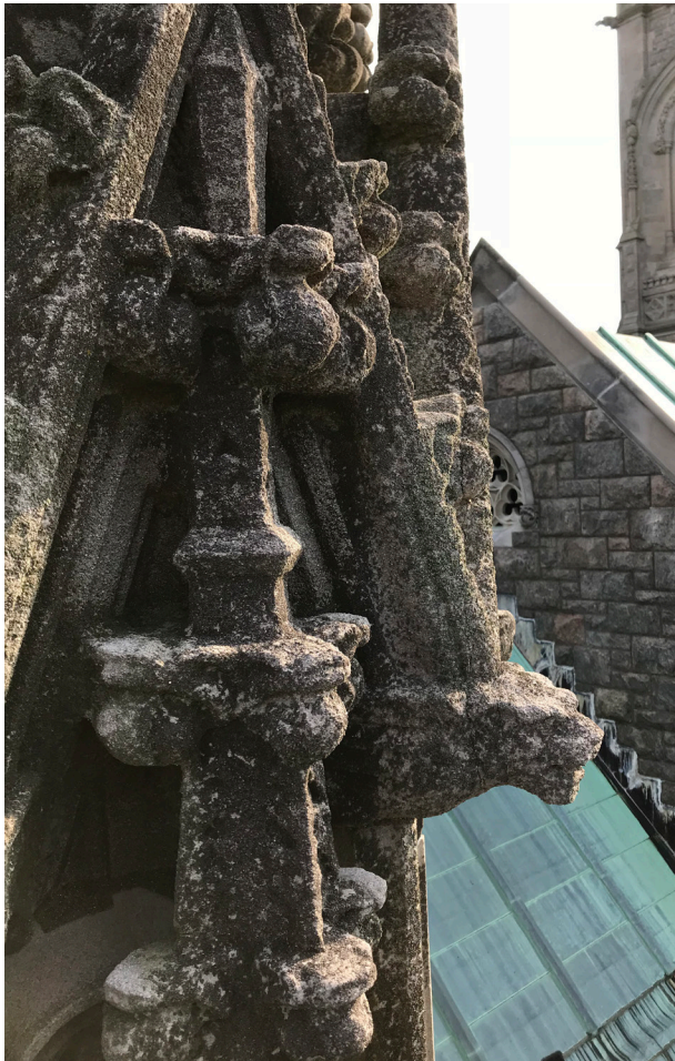
Finials on pinnacles have organic growth that should be removed followed by a careful inspection for loose elements to be re-installed with non-ferrous pins.
