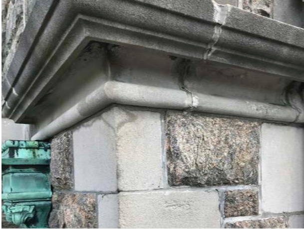
Cracks and spalls.
