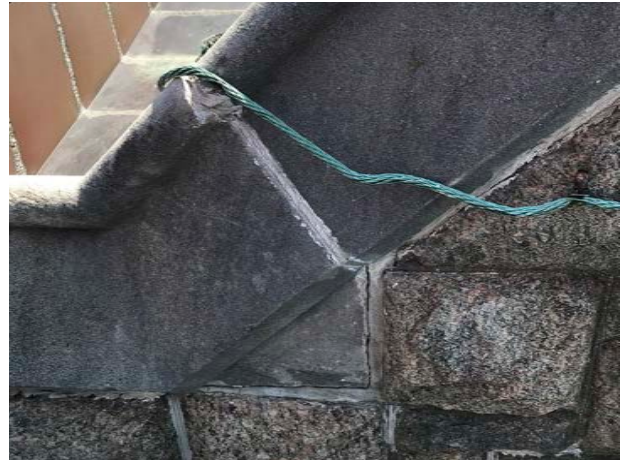
Stone movement, asbestos-containing caulk, open joints.
