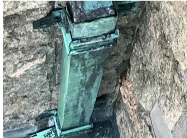
Old rain leader assembly at northwest corner of nave. Note: Some of these older assemblies were sleeved with new copper leaders during recent copper work.
