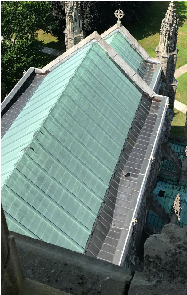
Newer replacement copper at nave roof valleys, and older copper roof at nave peak, possibly completed in 2004.
