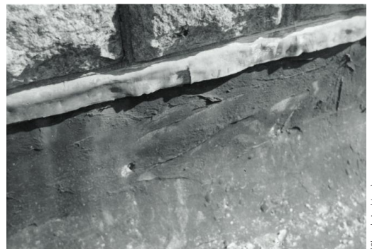
Waterproofing was already a problem in 1957 when this photo was taken.
