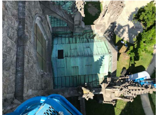
Original copper roof beyond its life expectancy.
