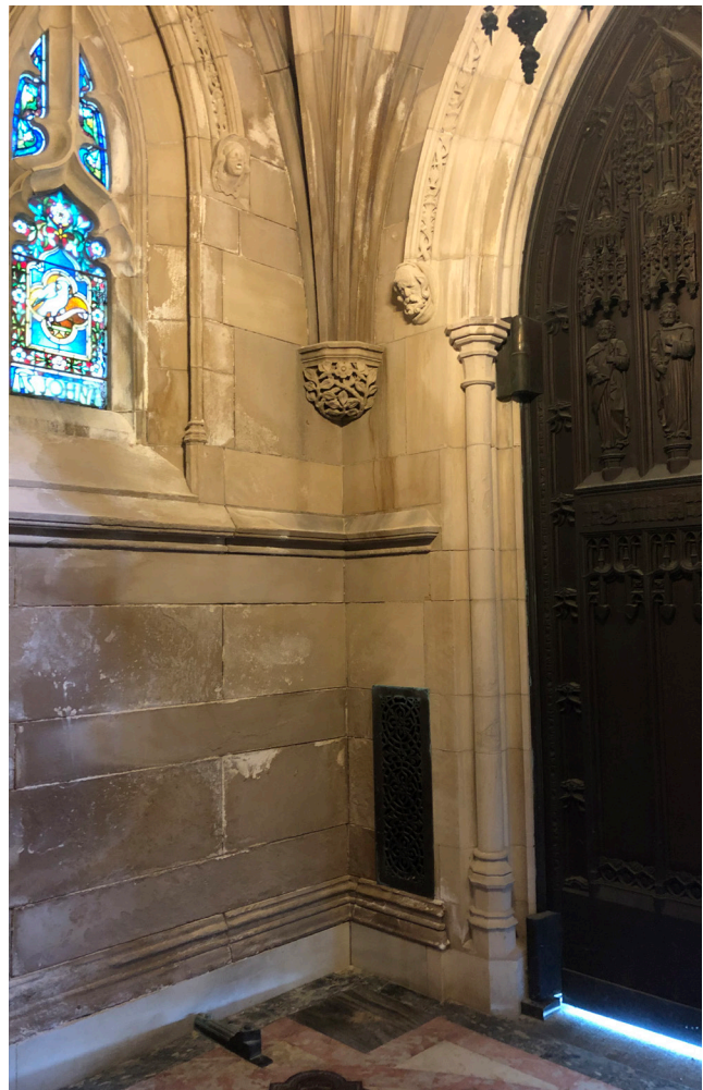
Southwest entry portico moisture damage.
