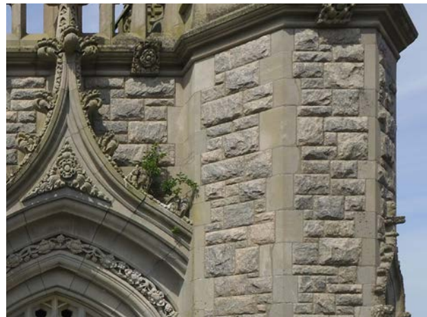
Remove small tree growing nearly at top of tower.
