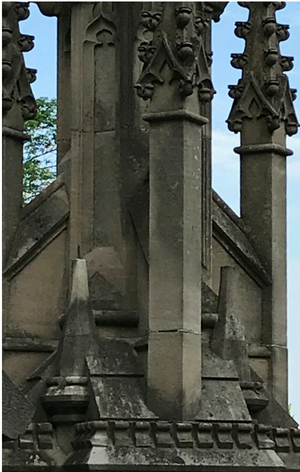
Missing and cracked finials and defective mortar joints.
