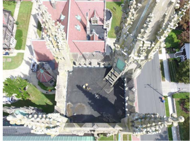
EPDM roof was patched during assessment and should be replaced.
