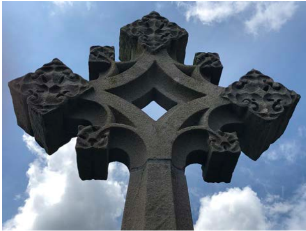
Stone cross at gable peak is cracked and loose.
