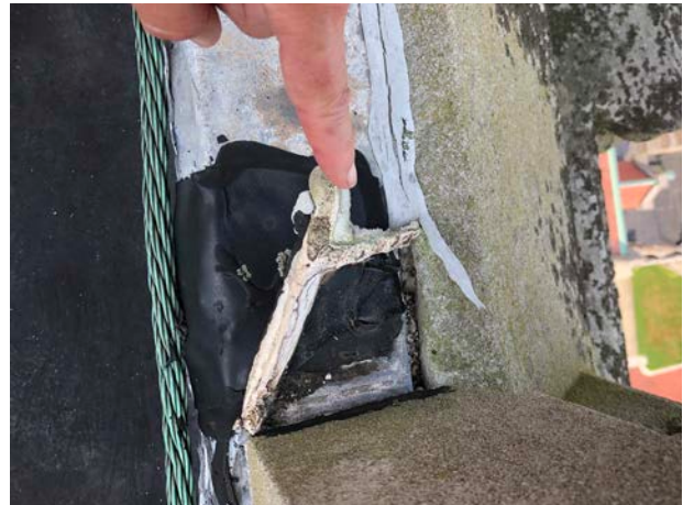
Tower roof has many failures of flashing and caulking on this roof. Note that white caulking was determined to be asbestos-containing.
