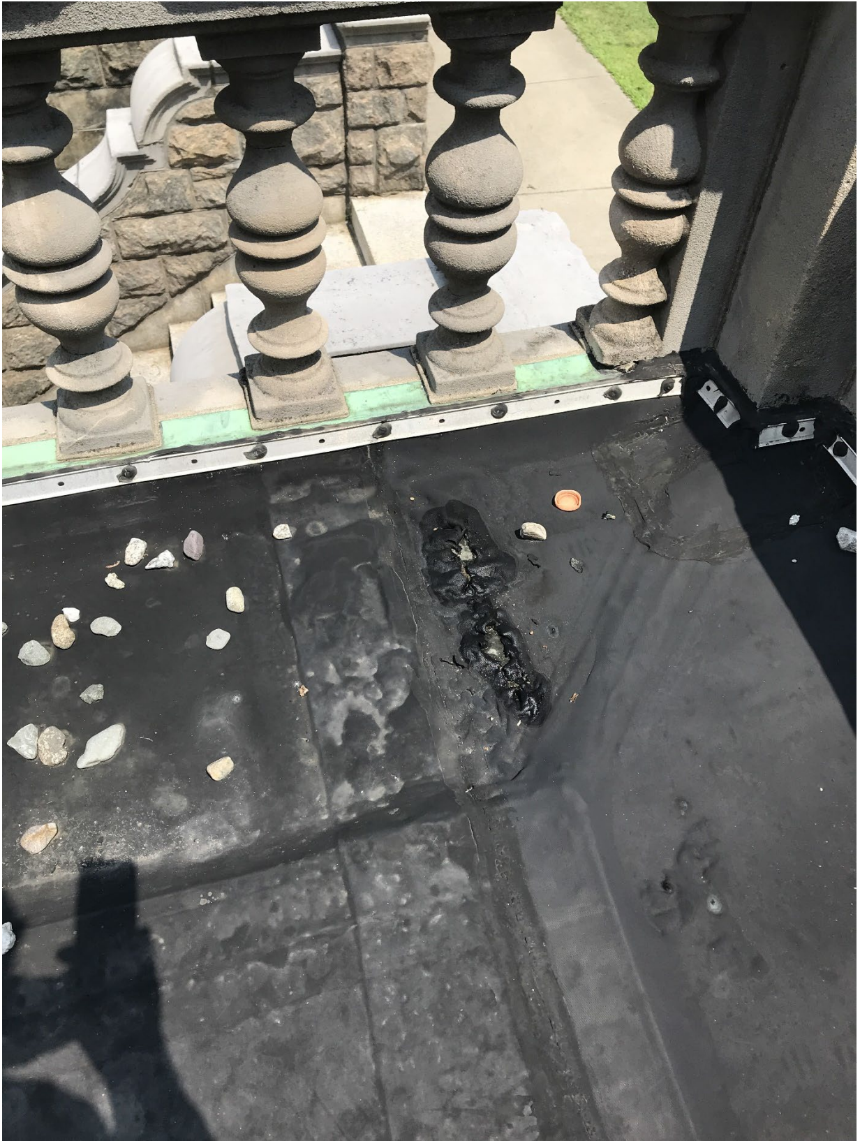
Figure 4 Detail view of deteriorated existing roof membrane
