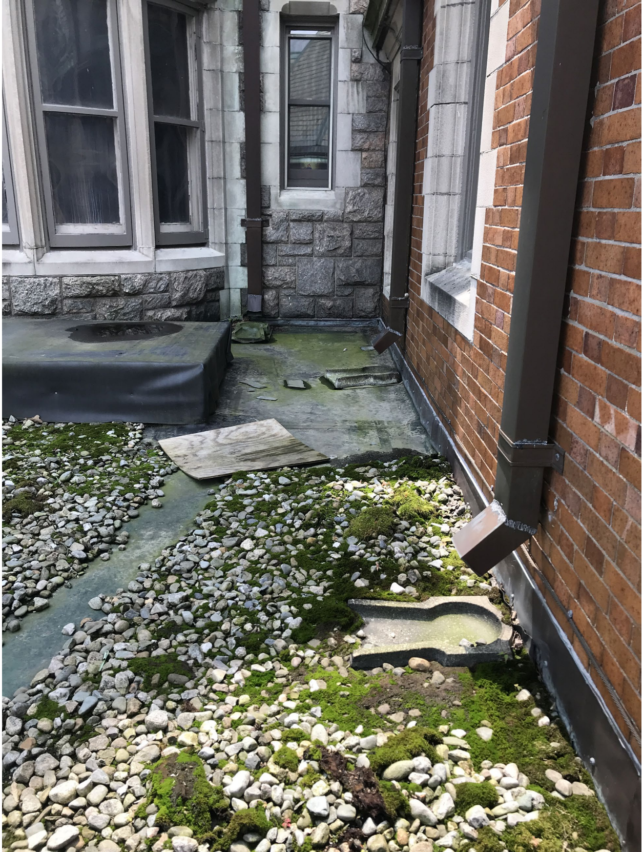
Figure 6 Organic growth and leaks plague the existing roof
