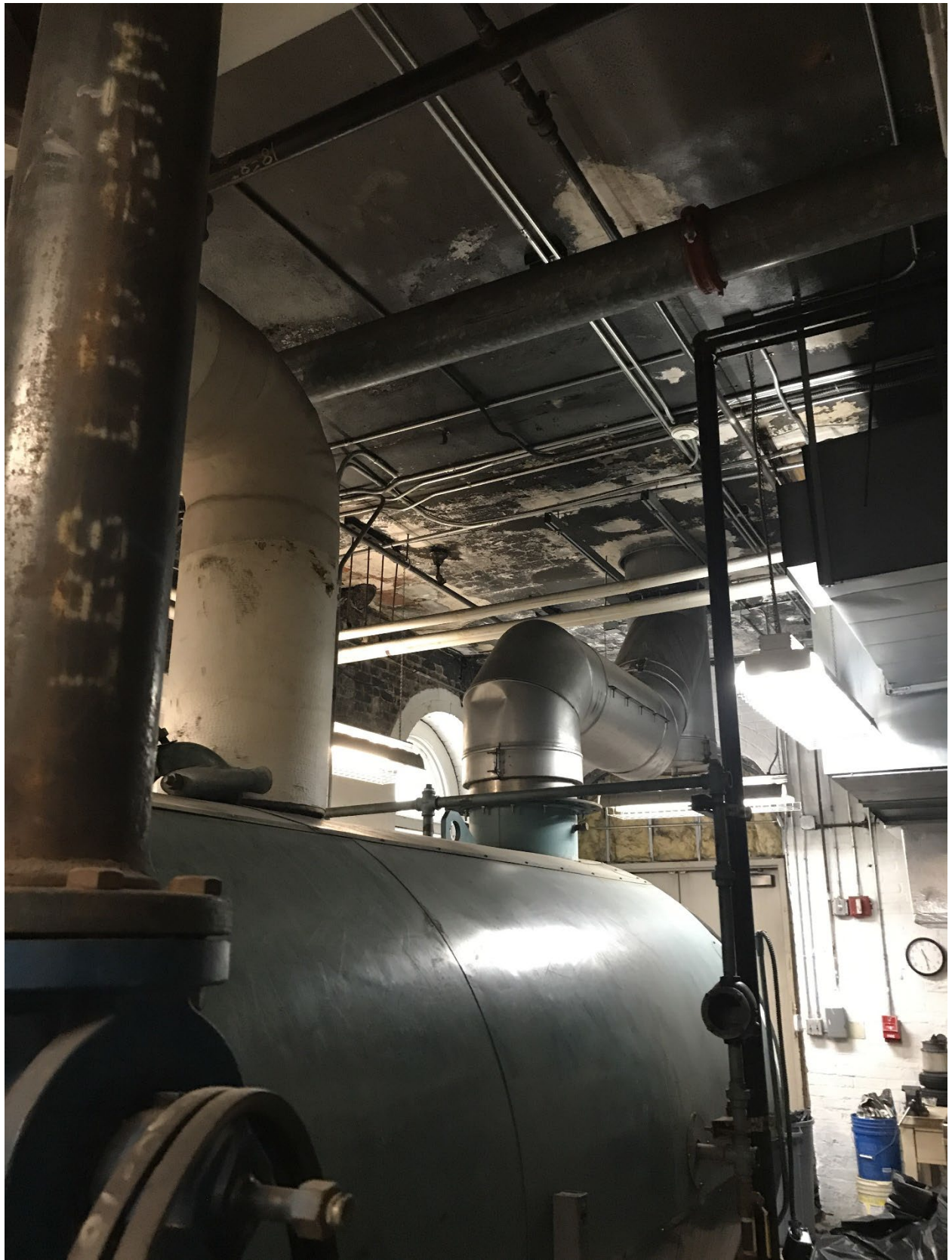
Figure 3 The existing roof leaks onto mechanical equipment in the boiler room below
