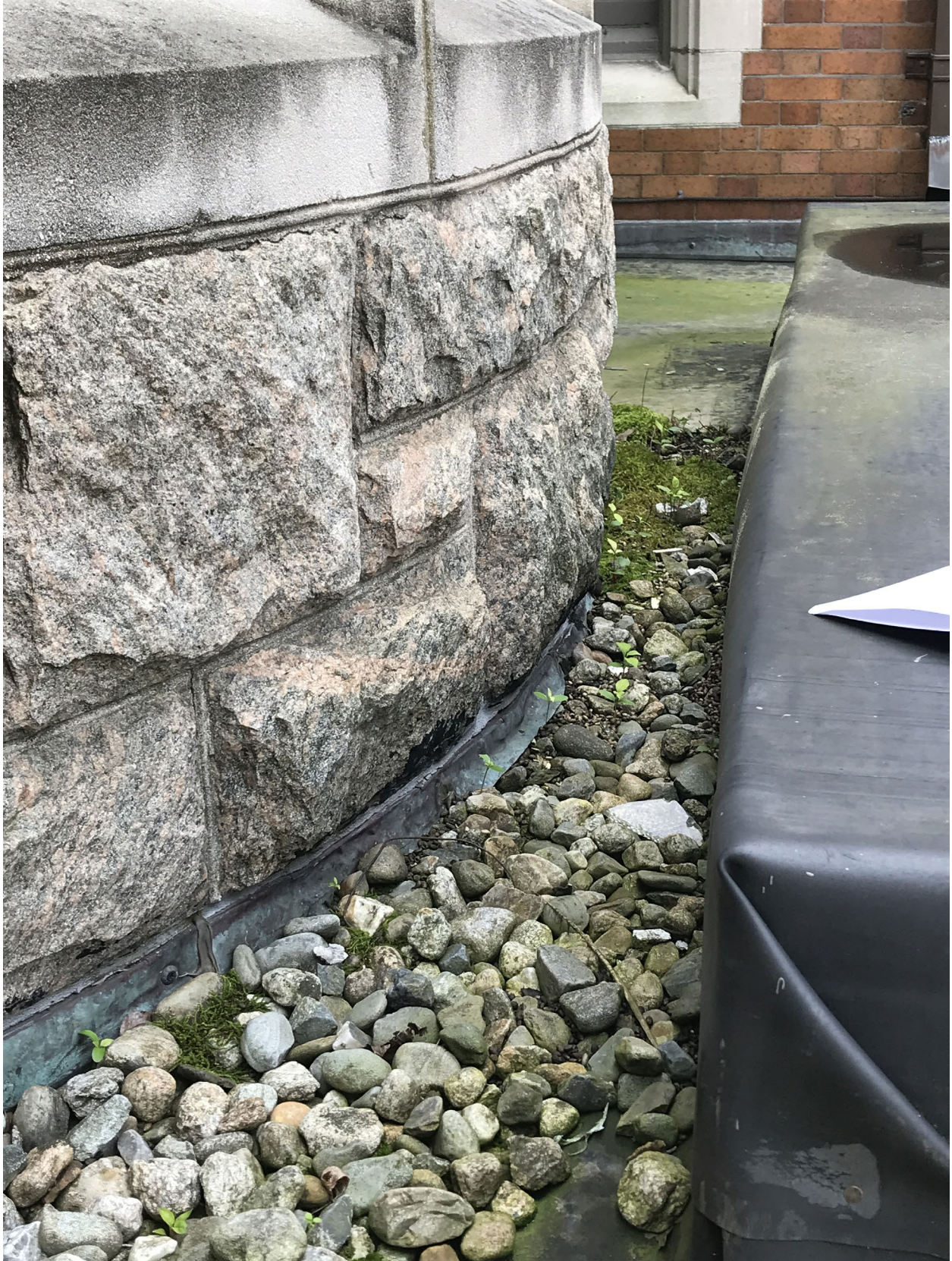
Figure 5 Perimete flashings need to be replaced with the roof
