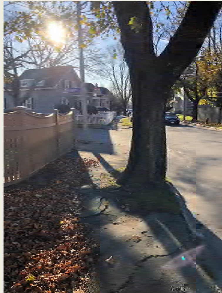
Sidewalk Surface in Below Average Condition on Spring St at Pleasant St
