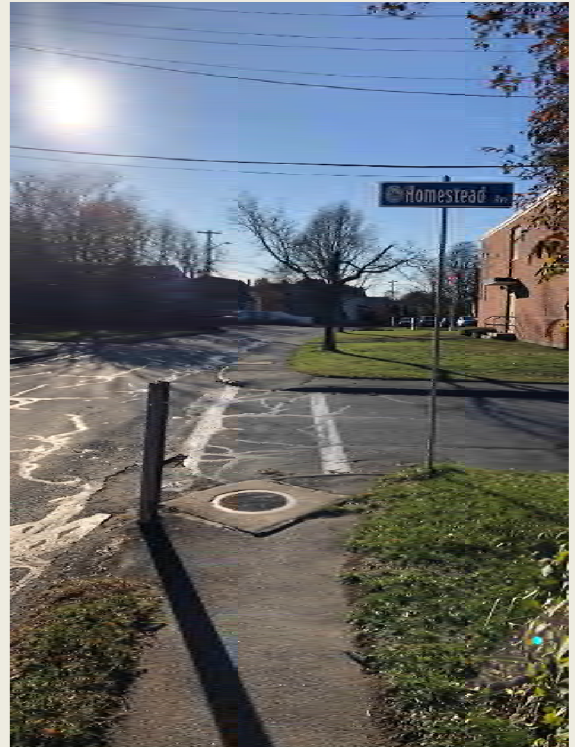
Non-ADA compliant crossing on Spring St at Homestead Ave
