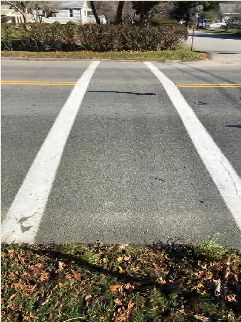
No curb ramp at Scoticut Neck Rd and Orchard St
