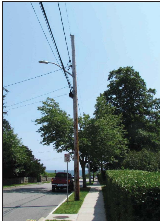
Figure 2: Existing Utility Pole at 6 Fort Street, Fairhaven, MA Which Would Host a Verizon Wireless SC Antenna
